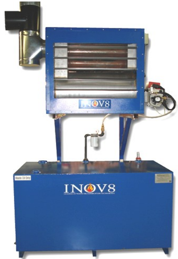
Photo shows a completed installation of a model F240 mounted on an INOV8 model T300 tank with a chimney, oil lines and gauge. Note that the brackets have been shortened.
